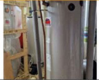
New Hot Water Cylinder installed – redundant ones still in place. Pipe connections not secure and bent. Pipe insulation not continuous. Poor installation.
