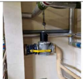
Plantroom gas solenoid valve and ECV located at rear of plantroom.
