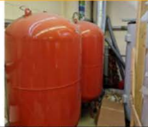
Expansion Vessels – Access restricted due to debris/waste material. Plantroom to be cleared.
